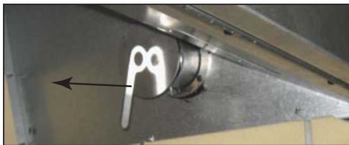
Figure 4 Outside Air Tube Opened
